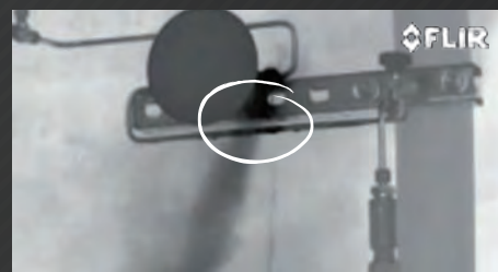
A LEAKING PRESSURE GAUGE
