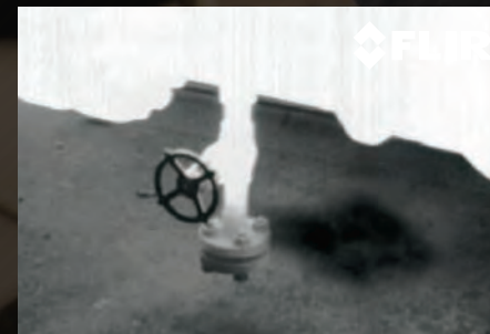
METHANE LEAK AT NATURAL GAS FACILITY SITE
