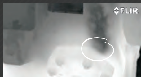
CAPTURED GAS LEAK
