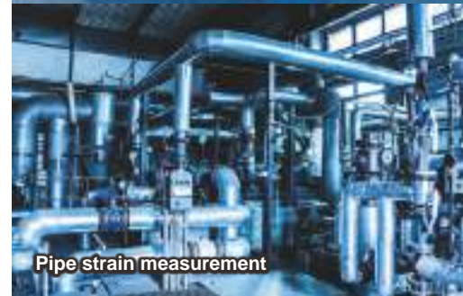
Brake and pipe strain measurement
