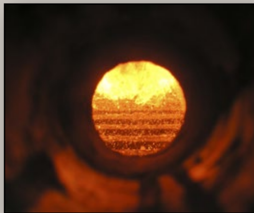
Interno camera di combustione Internal view of combustion chamber
