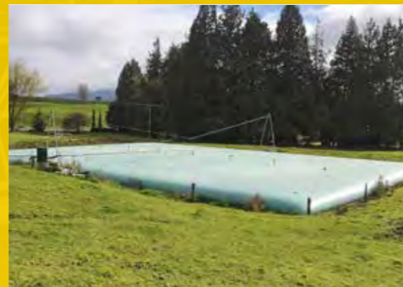
Waste water tank
