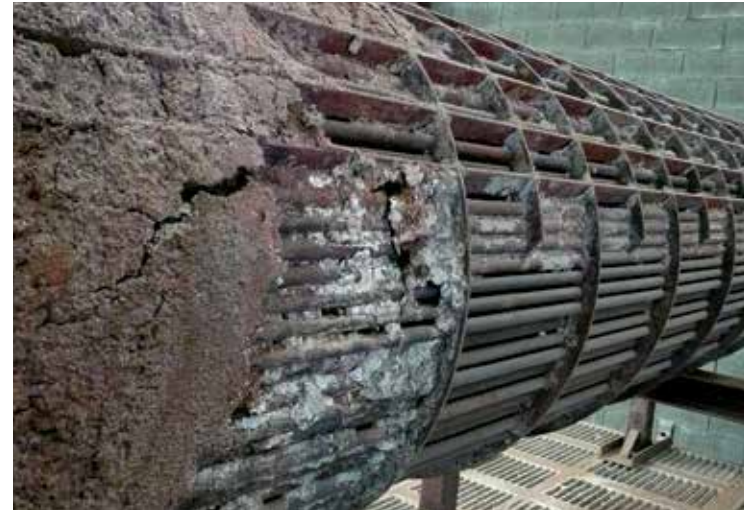
AFTER THERMAL CLEANING: 5% DUST, EASY TO REMOVE
