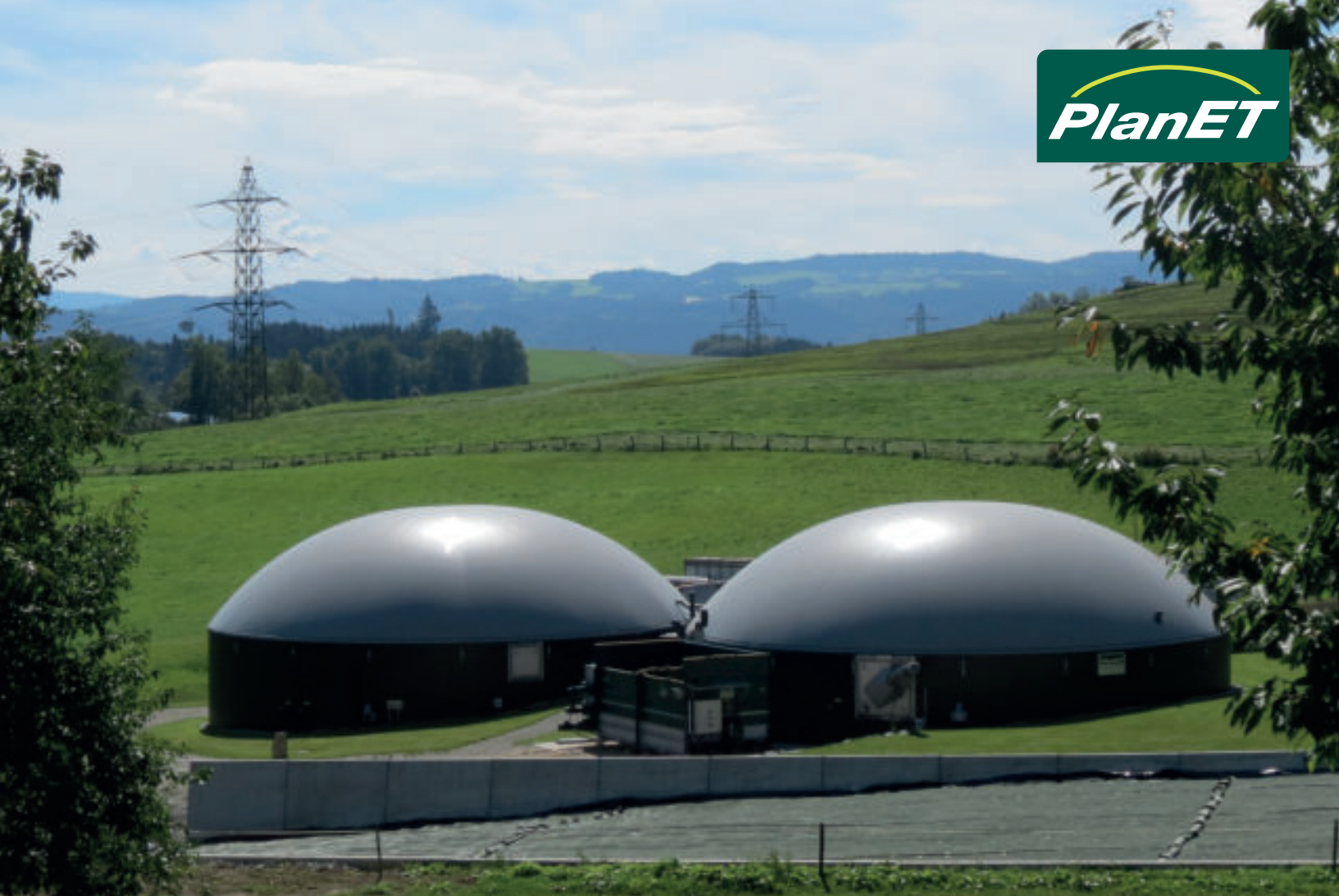
Installation de biogaz agricole
