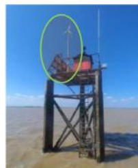
Green electricity supply : solar panel, wind turbine and battery
