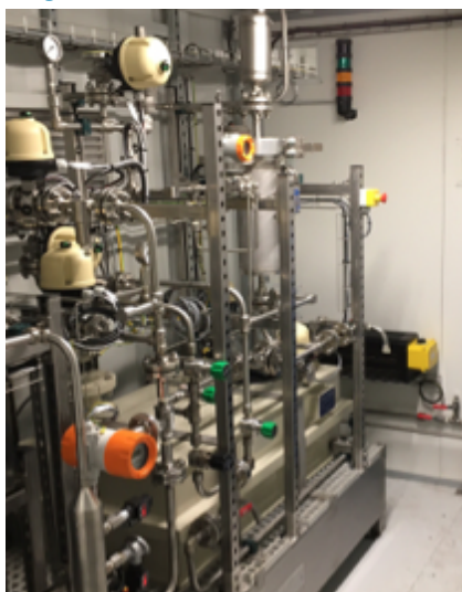
Industrial pilot plant for geothermal (designed and tested for 80°C and 40 bar)
